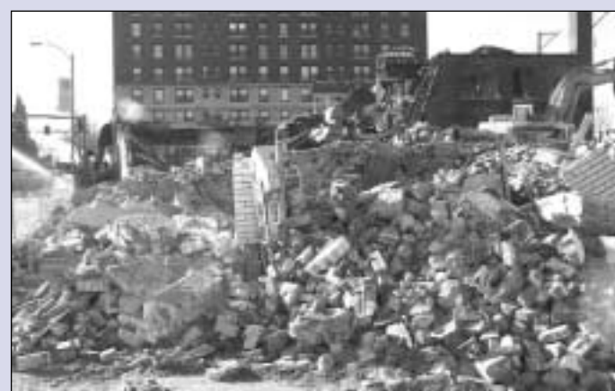
COMING DOWN: The end of February also brought the end of the Feathers and Marina buildings. The University hopes to attract a mixed-use building with ground-level retail at the site, located at the corner of Grand and Lindell boulevards. (Photo by Chris Waldvogel)
