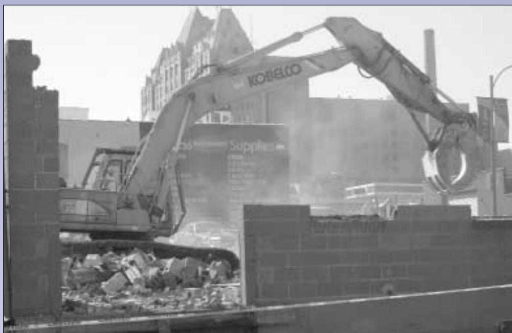
Below, a rendering of the Research Building Above, crews demolish a building at the corner of Grand Boulevard and LaSalle Street to make room for the proposed Research Building site. (Photo by Chris Waldvogel)
