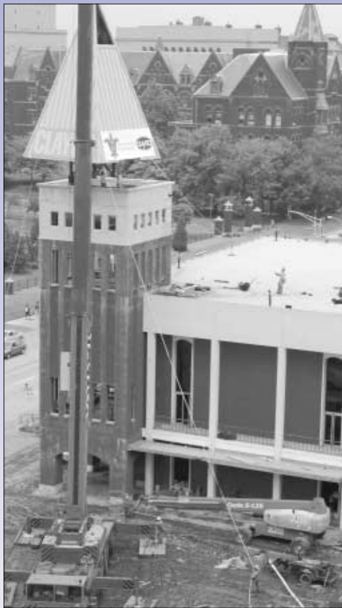
Crews from Clayco Construction Co. use a 100-plus-ton crane to lift a 32-foot, 22,000-pound steeple to the top of Busch Student Center's southwest corner on June 19. (Photo by Chris Waldvogel)
